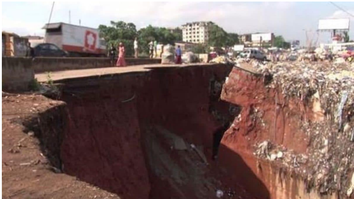
Figure 6. Erosion sweeps building in Awgbu, Anambra State, Nigeria. Photo Credit: Linus Unah.
