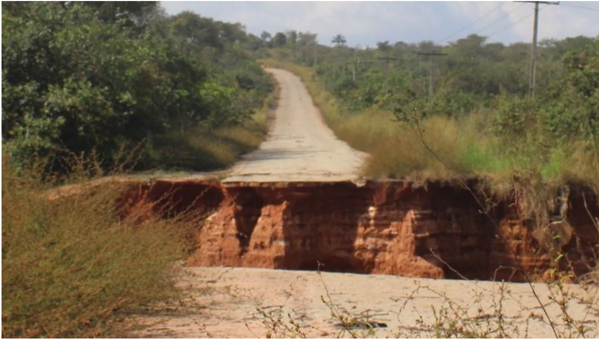
Figure 4. Erosion breaks inter-community road in Anambra, Nigeria. Photo Credit: Linus Unah.
